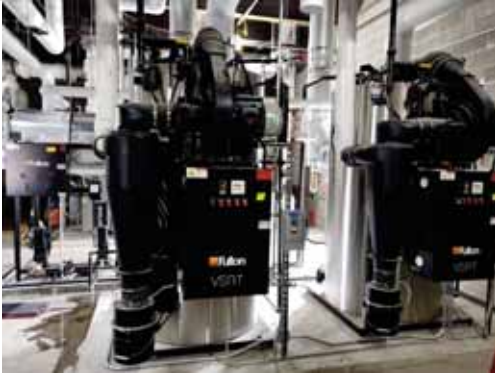
(2) Fulton VSRT 40 boilers used for the Hutchinson Health Care's humidification
