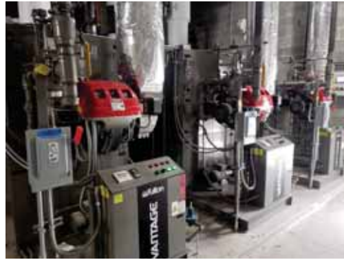
(3) Fulton Vantage 3000 Gas/oil used for Hutchinson Health Care's heating needs.
