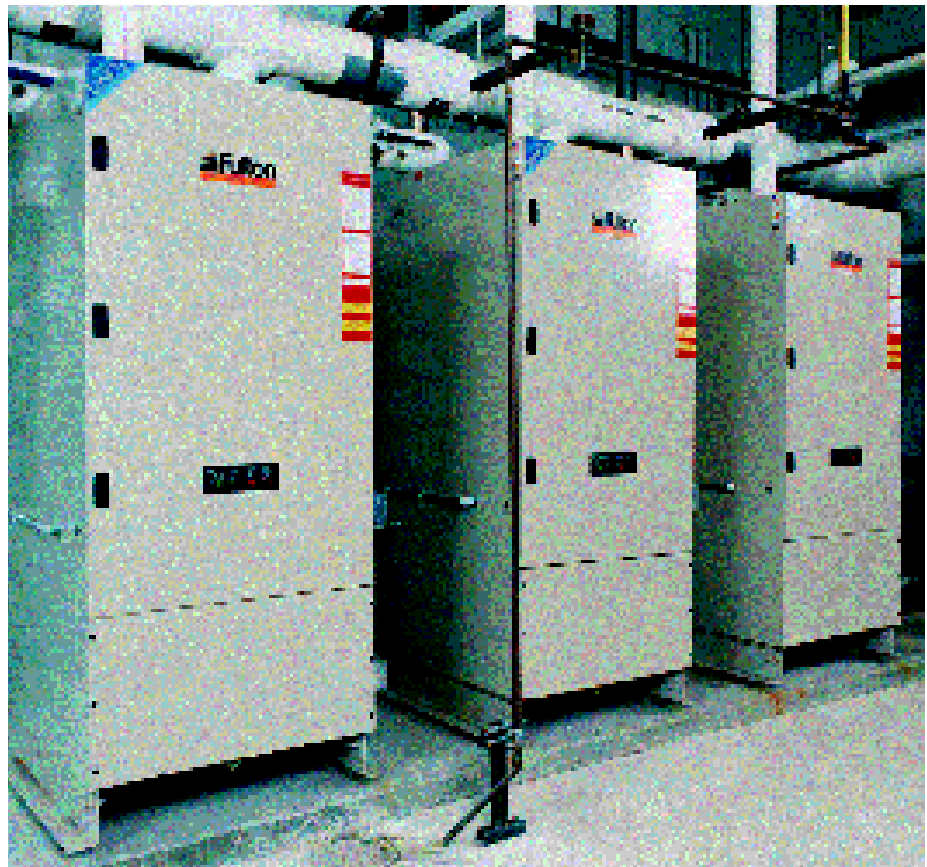
An array of three Fulton PHW750 units replaced much larger boilers with power burners in Maintenance Hanger building 400.
