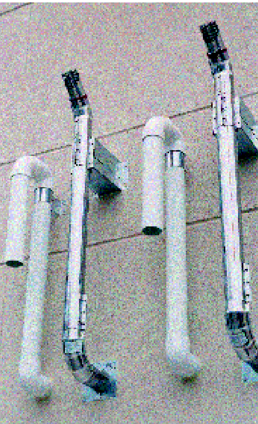
Intake and exhaust stacks on the exterior wall serve two Fulton PHW1000 boilers
